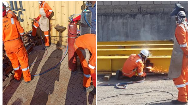
Figure 4. Sparks Near Acetylene and Diesel
